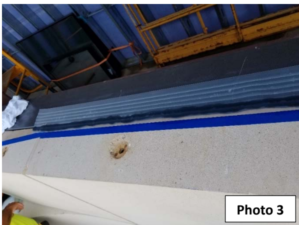
Membrane set in place on one side of joint and ready for tooling.
