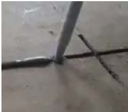
Joint Overfill (crown)
